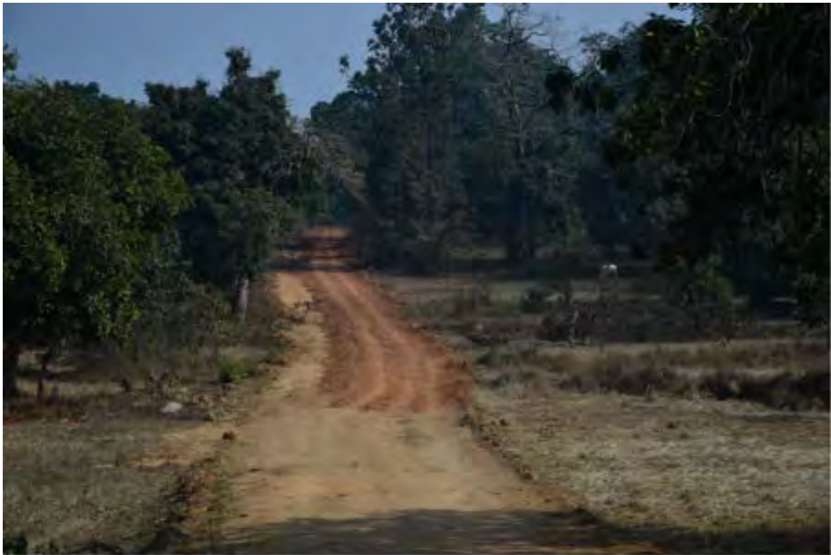
Figure 13: Road at Burji village, this road is being laid from Gangaloor to Nelasnar
