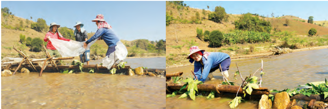
Women work together to build a small dam in Huay Lu Luang stream
