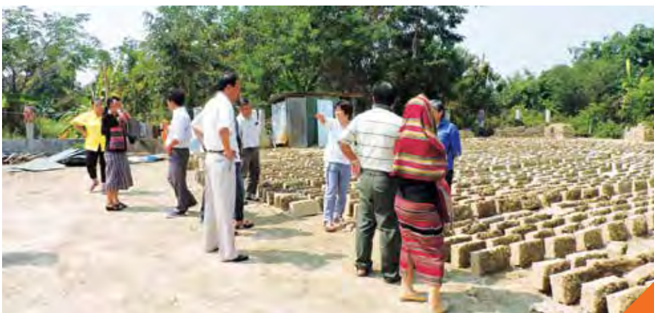
❖ The Executive Council paying a visit to the building site of the AIPP Eco-office in February 2016. Photo Credit: AIPP
